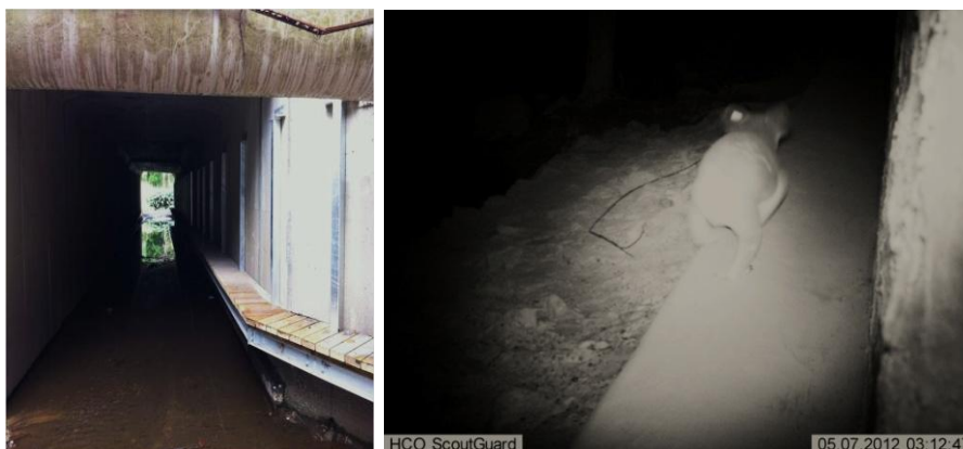
Figure 2: The left hand panel shows the design and layout of a 'safe passage' under a major road. Note the raised animal walkway on the right hand side of the tunnel. The Right hand side panel (infrared image) shows a koala using the raised walkway through this tunnel to safely move from one side of the road to the other at night.
